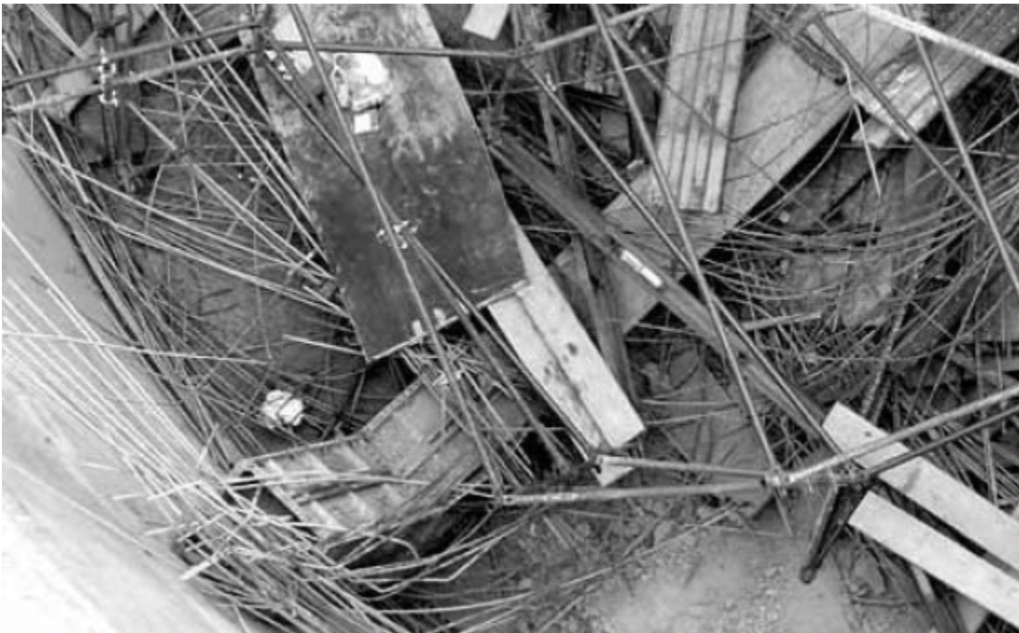
Tower Collapse in Lake Cargelligo 22 October 2002, two killed.
